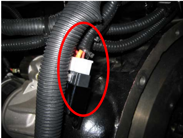
Incorrect Orientation Water can pool in connector
