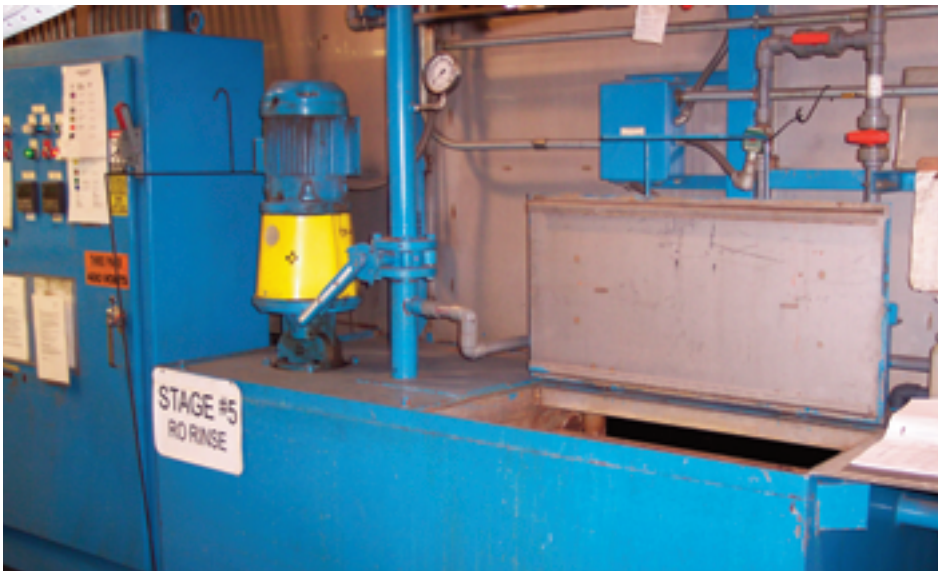
FIGURE 2 Instead of dumping and refilling all five tanks of the pretreatment system for DeWys Manufacturing's powder coating system with fresh water, the manufacturing team now fills the first tank with fresh water and backflows the rest of the tanks, dumping the dirtiest water and using fresh water to top off the other tanks if necessary.
